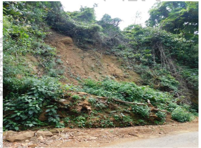
Photo 16: Road cut failure near Kursi.
