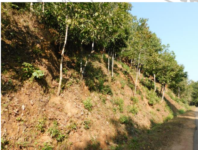
Photo 17: Extensive cut failure near Kansur.
