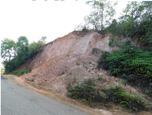
Photo 9: Road cut failure along Herur-Golmakki road section.
