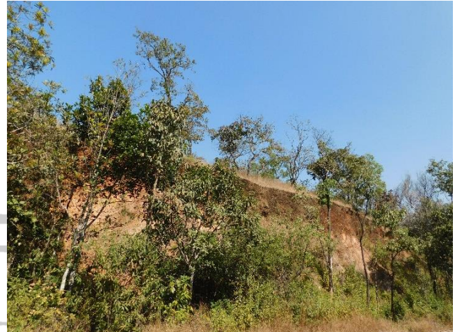
Photo 8: Old landslide scar along Sirsi-Siddapur road section.
