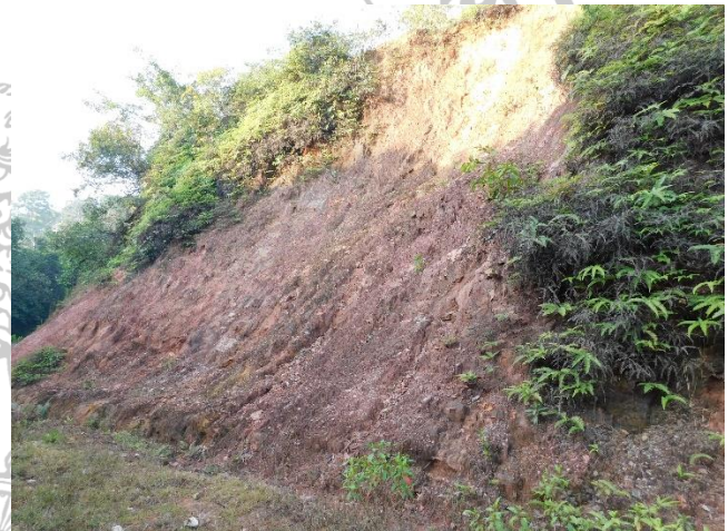
Photo 10: Extensive slope cut along Ammenhalli-Marur road section.
